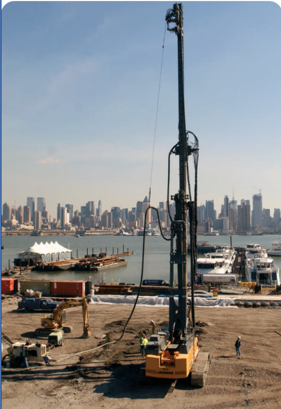
View of Menard's CMC operation showing grout delivery, pumping and drilling — directly across the Hudson River from midtown Manhattan.
