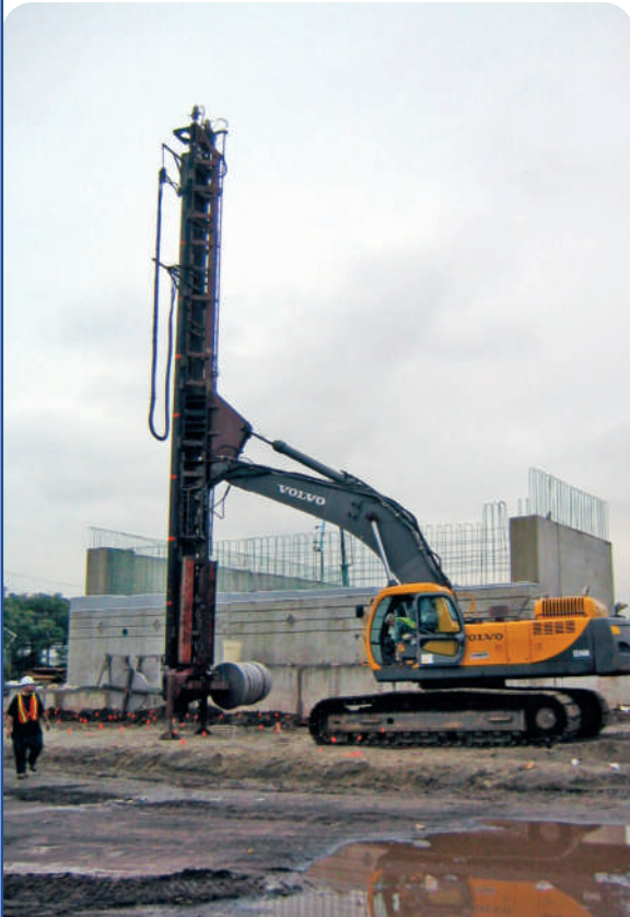
Menard installed 9,000 Prefabricated Vertical Drains (Wick Drains) to depths of up to 30 feet.
