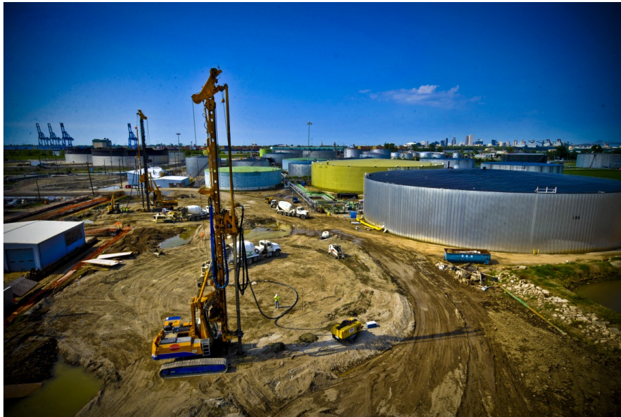
Private Client - Marrero Tanks
